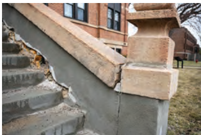
After many years of use, the Old Main stairway is crumbling and unsafe.
