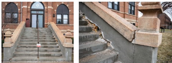
After many years of use, the Old Main stairway is crumbling. To address both safety and aesthetic concerns, it needs to be replaced.
